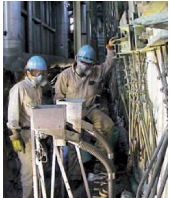
Two SpiraLoad™ units in operation
