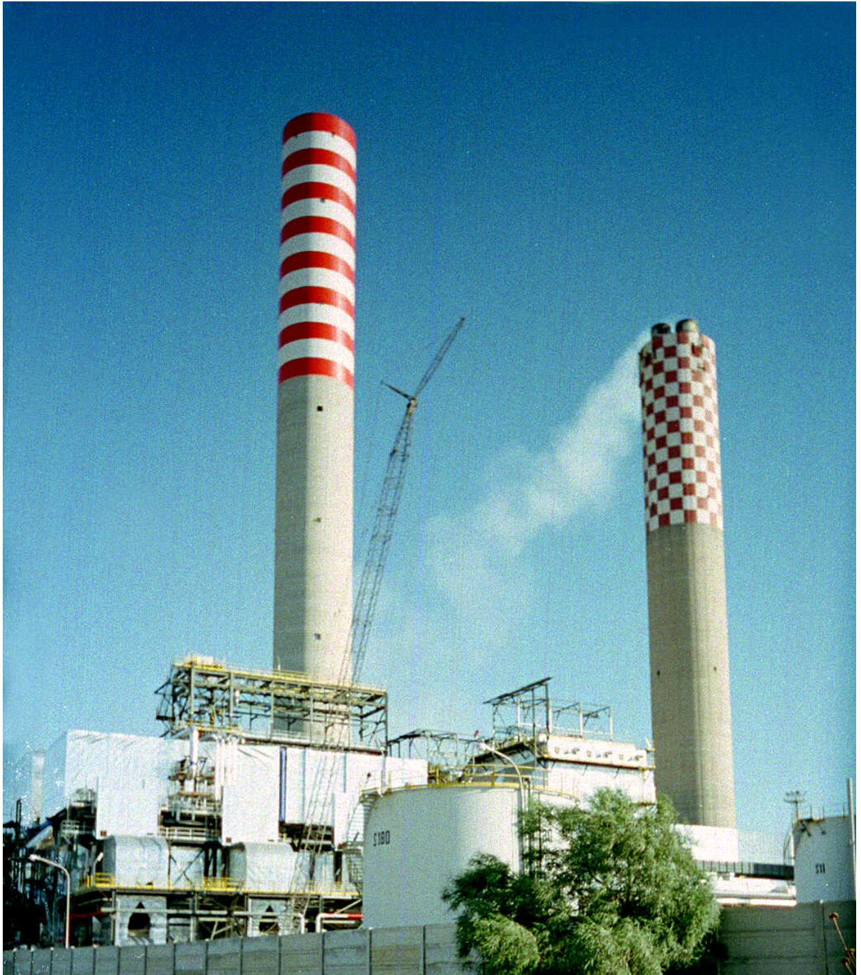
Fig. 2: The SNOX plant treating the flue gas from three boilers burning high sulphur petroleum coke at the Agip Petroli SpA refinery in Gela, Sicily, Italy. The banded stack seen on the left emits 1,000,000 Nm 3 /h of SNOX treated flue gas. The chequered stack seen on the right emits flue gas from the 4th boiler before it was connected to the SNOX plant.
