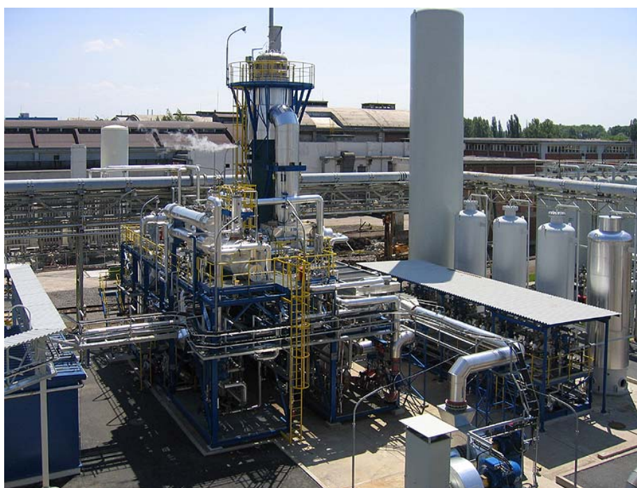
Figure 12: Plant in operation June 2005
